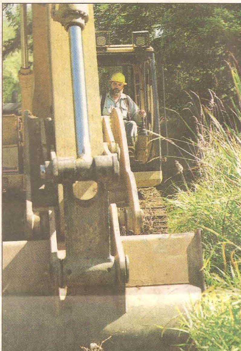
DAMIAN MULINIX — East Oregonian Publishing Group Leo Kuntz, owner of Nehalem Marine Manufacturing , uses a track hoe to remove land mass from along the banks of the river, allowing the water to come into the wetlands as the water levels rise.
