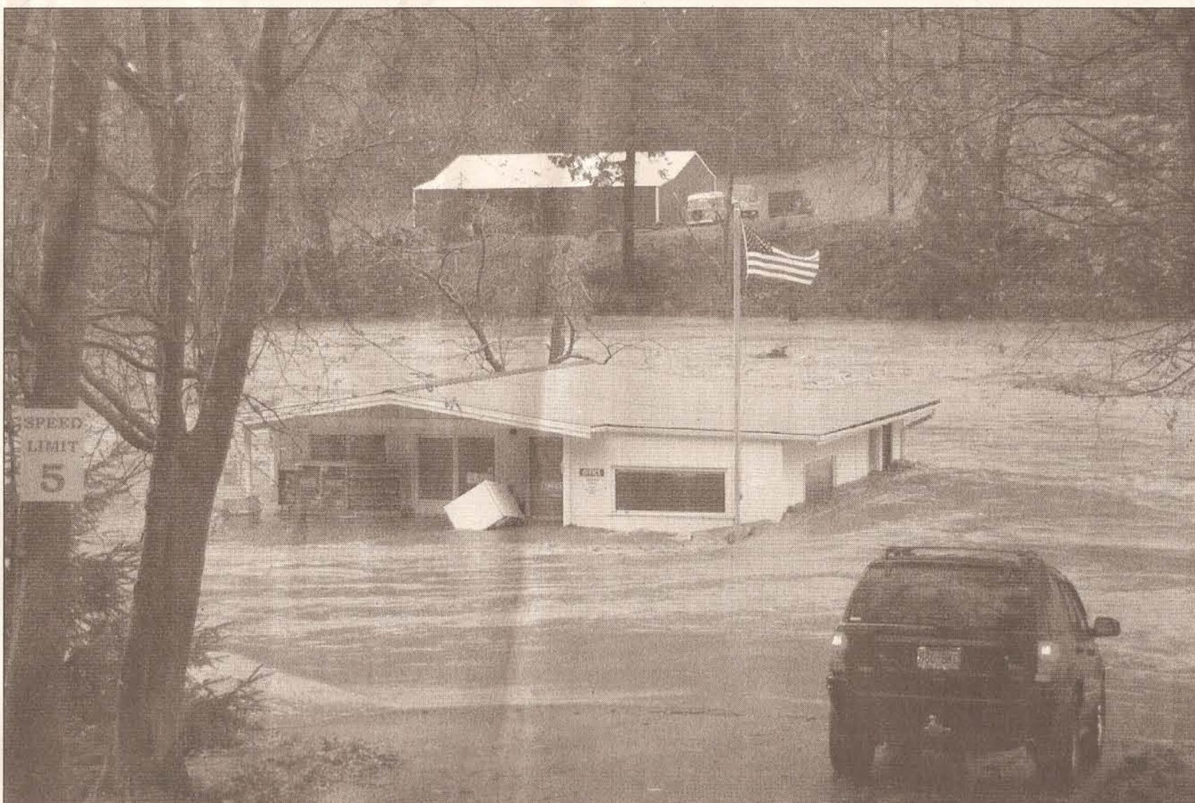
Raging waters of the Wilson River tear through the office and parking area at the Wilson River RV Park Monday, Nov. 6. The office was ripped off its foundation and washed several feet downstream.
