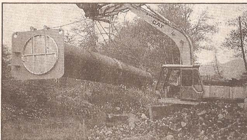
Leo Kuntz installs a new tidegate, which will help juvenile fish habitat by allowing fish movement. Many tidegates in the county from the early '50s are being replaced.
